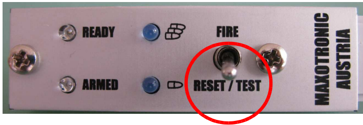
Figure 1: Control unit ready for testing
