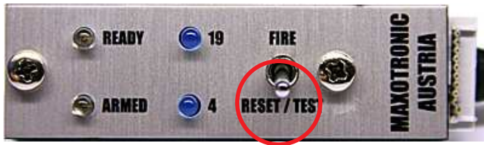
Figure 1: Control unit ready for testing
