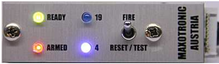
Figure 5: Control unit after second operation
